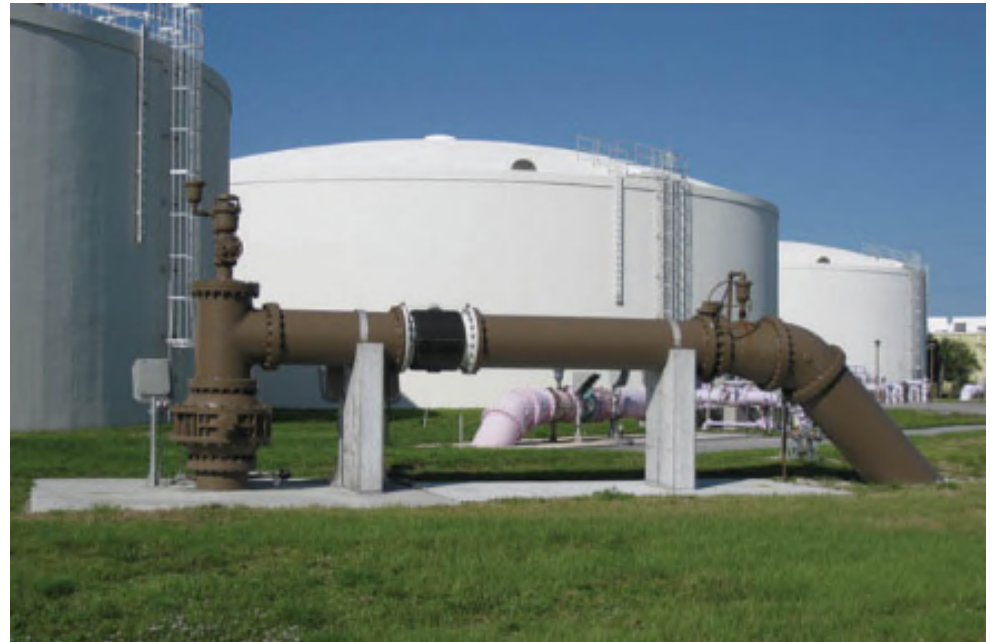
Deep Injection Well at Delray Beach South Central Facility
