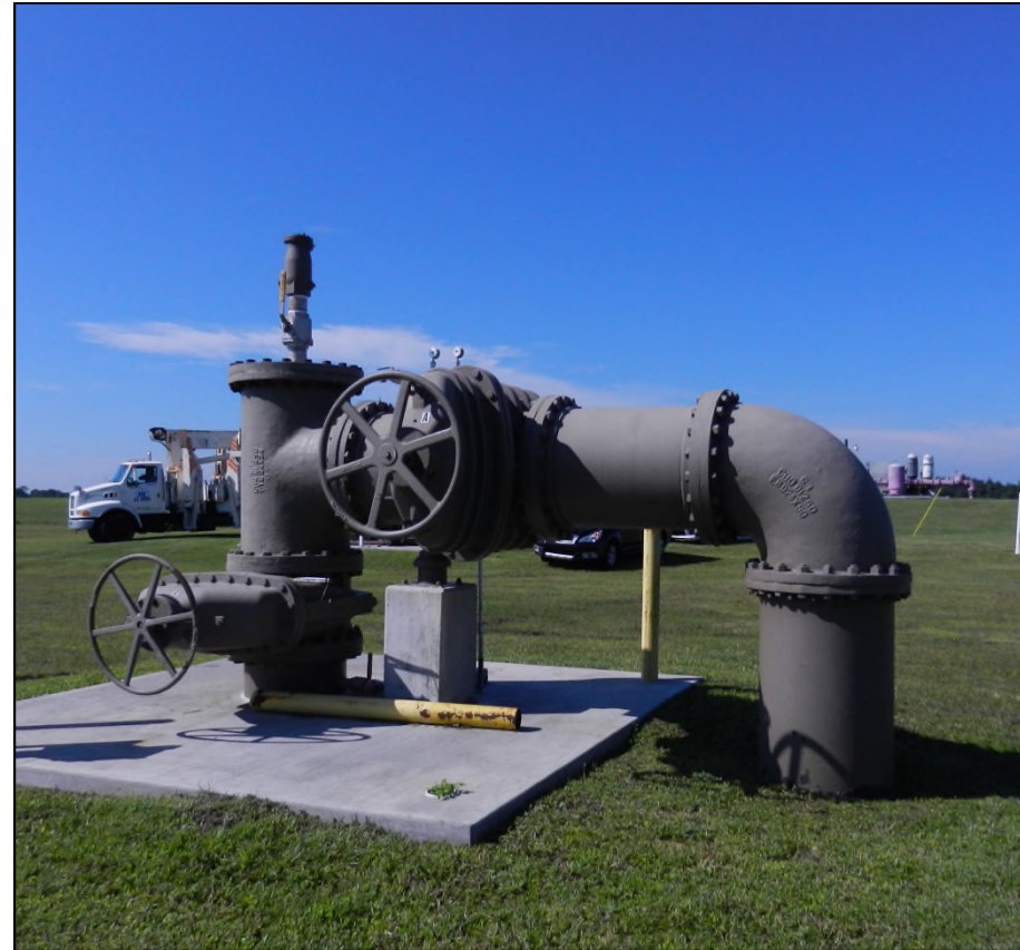
Deep Injection Well at the Okeechobee Utility Authority, since 2009
