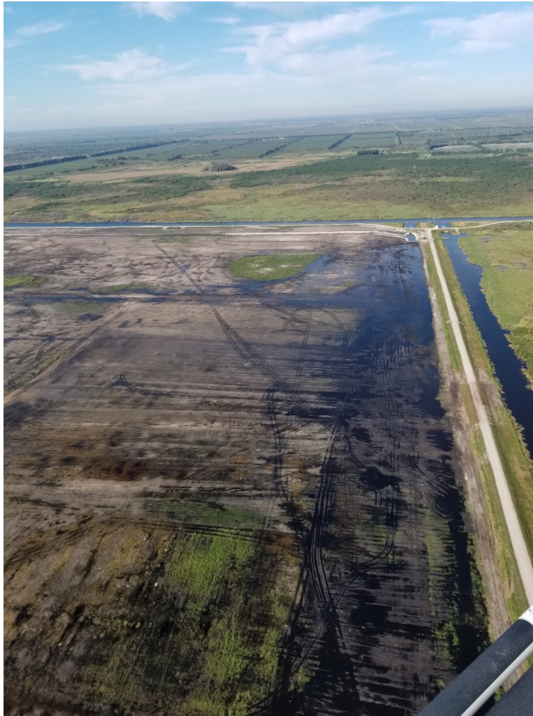
Figure 5A-9. STA-5/6 Internal Improvements. View of earthwork in Cell 2A facing west (G-342C). (Photo by SFWMD in November 2019.)
