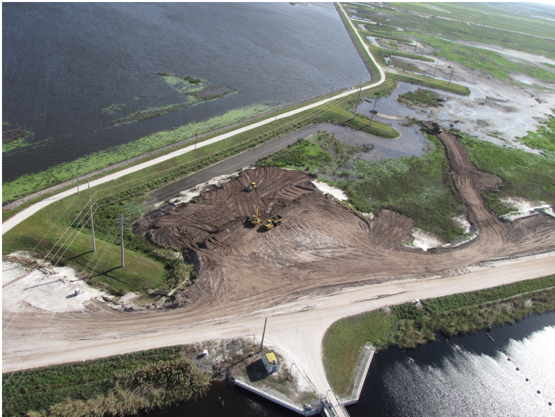
Figure 5A-4. View of fill material staging area at the Northwest corner of STA-1E Cell 7 facing East. Cells 5 and 7 are undergoing regrade. (Photo by SFWMD in 2020.)
