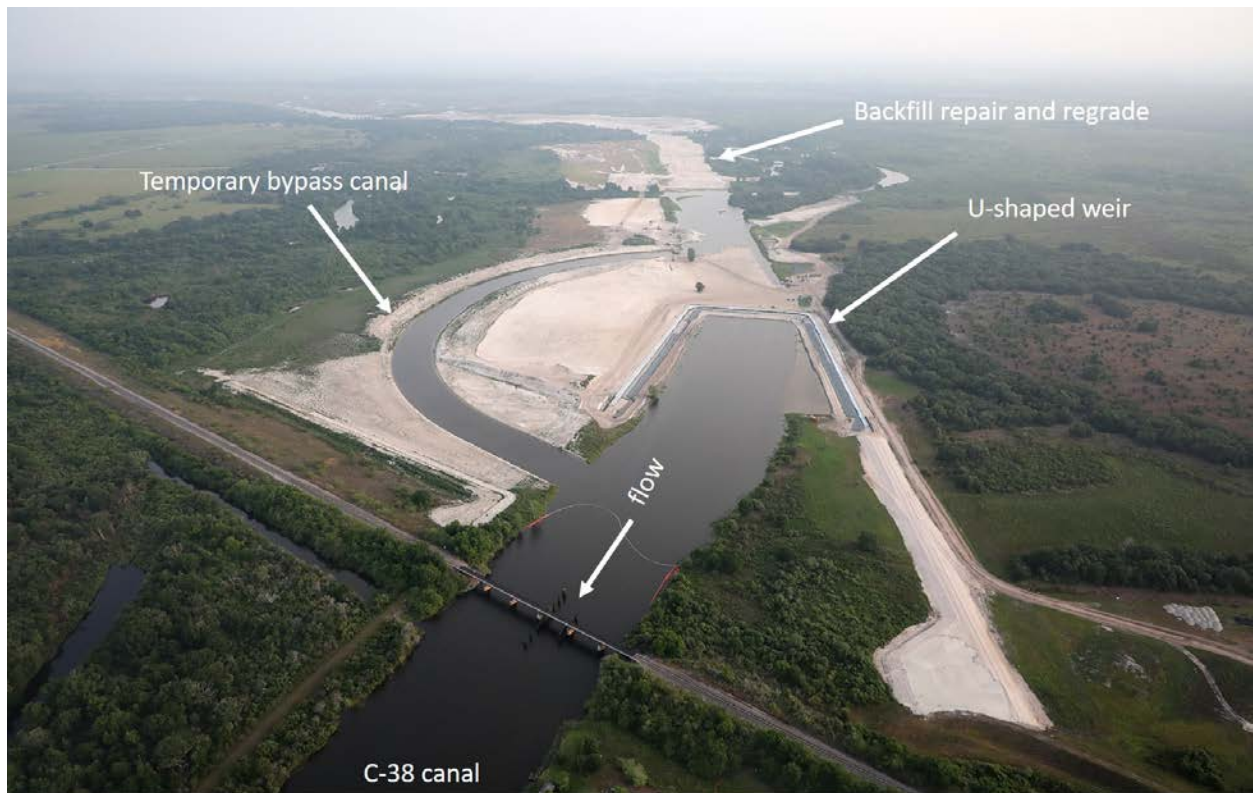
Figure 9-4 KRRP Reach 3 backfill repair work and S-69 weir construction. Photo by Brent Anderson on February 13, 2020.
