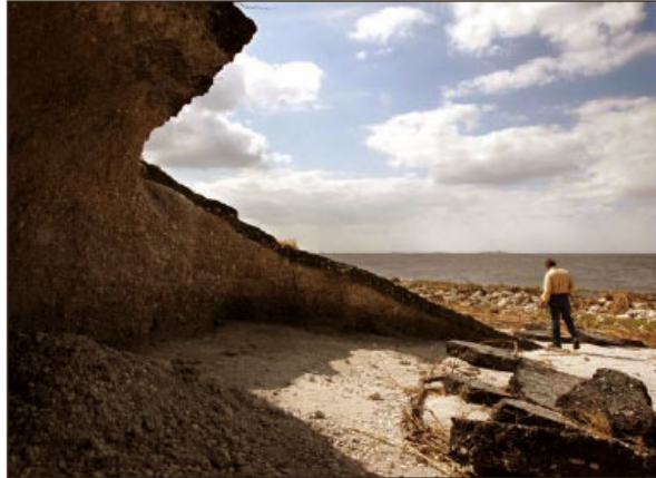
Figure 2-13. Wave erosion damage to the Herbert Hoover Dike from Hurricane Wilma (Bromwell et al., 2006).
