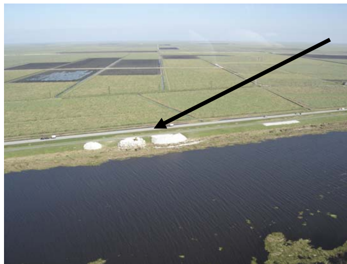
Figure 48. Lake Okeechobee levee damage from Hurricane Wilma (photo by SFWMD).
