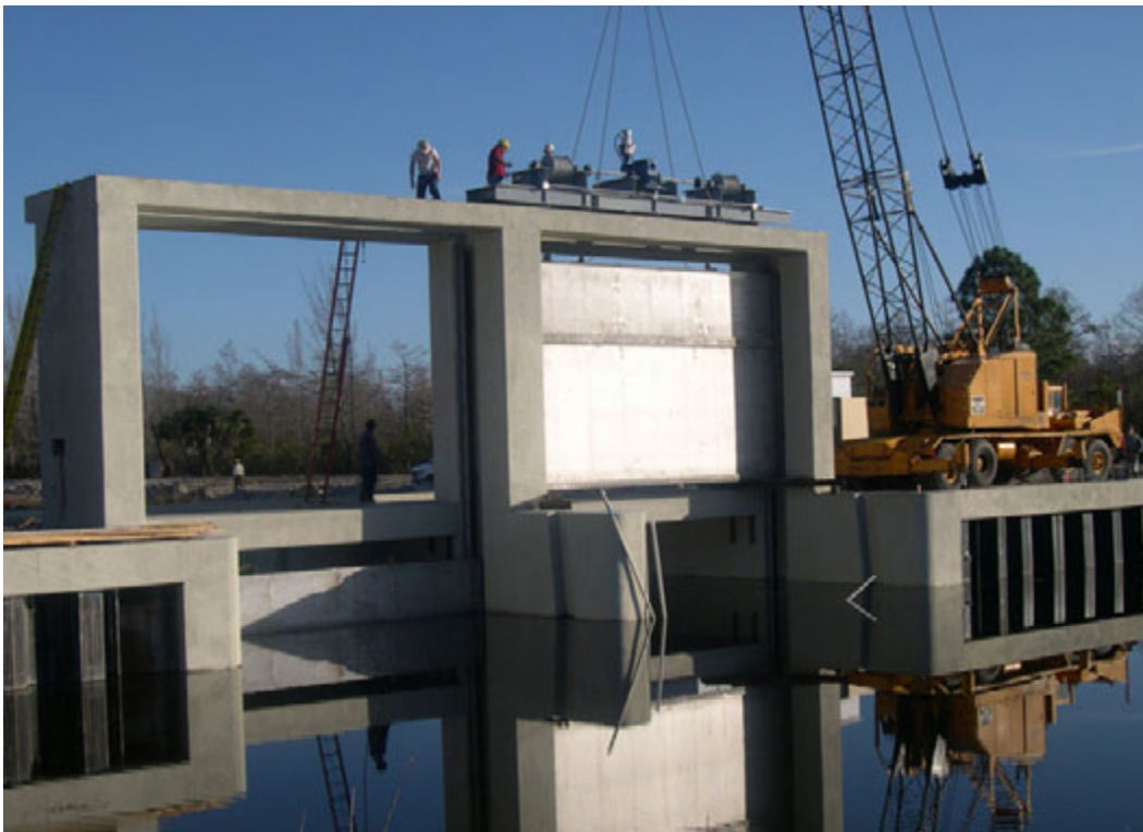
Figure 5-7. G-160 Loxahatchee Slough water control structure (source: SFWMD).
